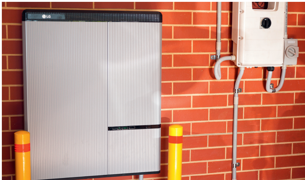
LG lithium ion home battery and Solar Edge inverter solar panel system for domestic power storage installed in home garage. Adelaide, South Australia
